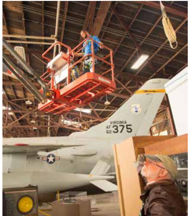
Deputy Chairman Dave Murray watches as technicians from Lesser Electric prepare to install a new light fixture
